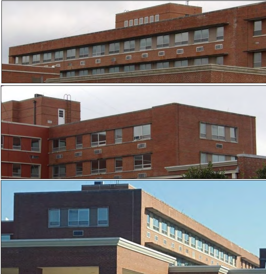
Photo 33: Detail of the Third and Fourth Stories of the Original Core of the Vidant Beaufort Hospital, South Elevation (Top), Northwest Oblique (Center) and Southwest Oblique (Bottom).
