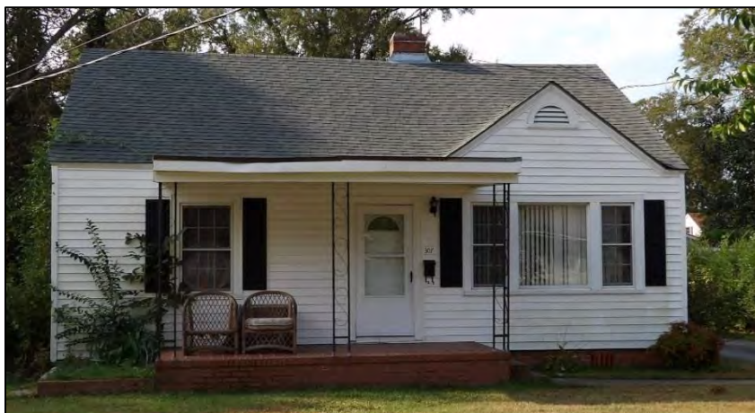
Photo 57: 307 E. 13 th Street. Note the replacement vinyl windows with an applied vinyl grill giving the appearance of six-over-six windows.
