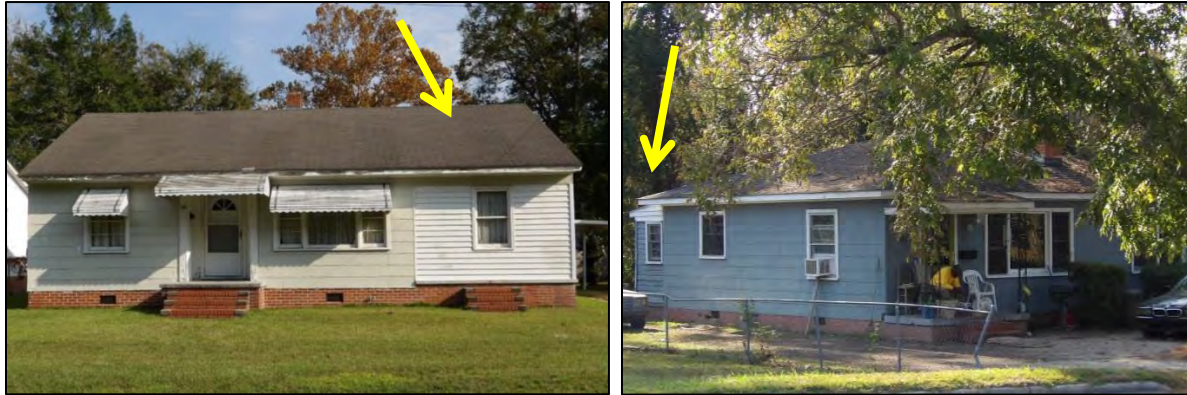
Photo 60: Example of an Enclosed/Altered Side Porch at 310 E. 13 th Street (Left) and a Rear Addition at 305 E. 15 th Street (Right), Noted by Yellow Arrows.
